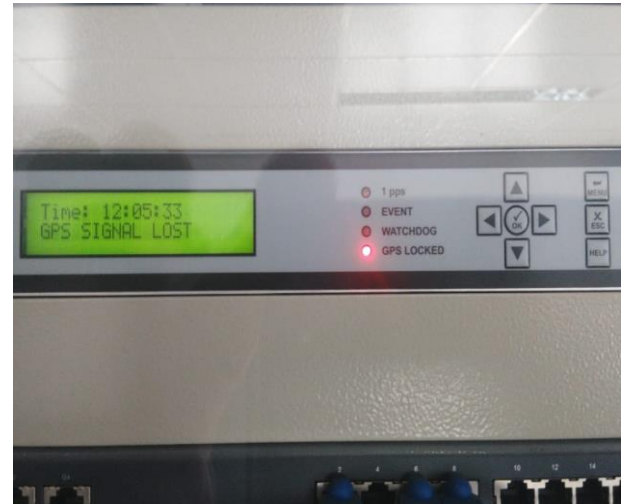
Fig. 5. GPS Isolated from SCADA
